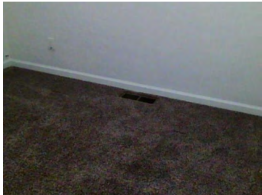
HEAT & DUCT CHECK.jpg
